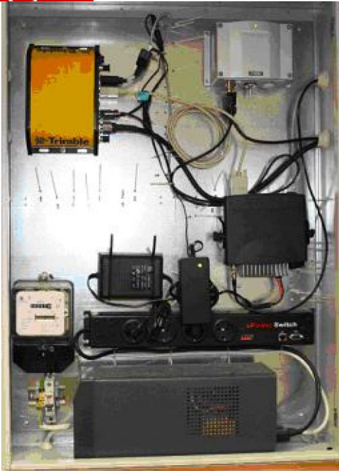
Fig. 1. LitPOS station with Trimble NetRS receiver
