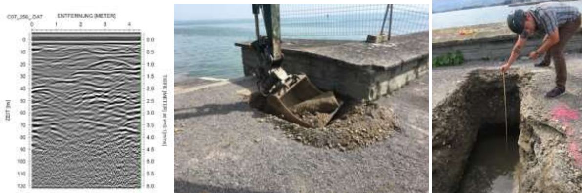
Fig. 12): The Profile C7 has a distinct hyperbola (picture left). The excavation brings out a large stone block (middle picture). The remaining excavated material consists of round stones of 3 - 5 cm diameter with little finely granulated material. The water flows immediately (picture right).
