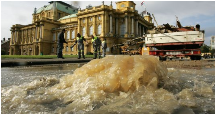
Figure 6. Water pipe perforated during survey activities for underground garage in Zagreb city centre – October 2010
