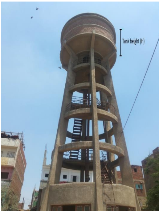
Figure 2 water storage tank at Meet El- Qurashy
