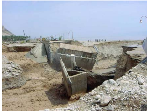
Figure 1. The Arugot Bridge during the May 2001 flood; the bridge collapsed as a result of a headcut backward migration along the stream channel.
