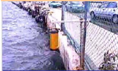
Radar sensor (f=24,125 GHz, p=25mW) was installed at Haifa port in 2001 and at the Ashdod port in 2004
