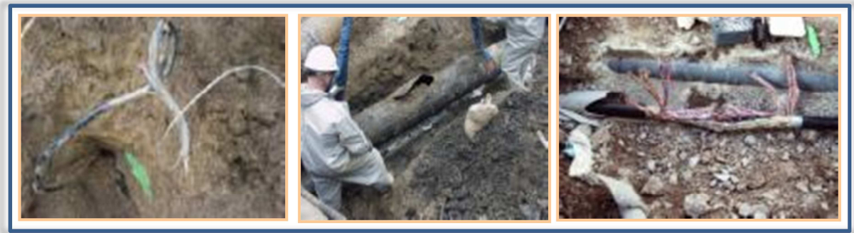
Figure 1: Damage utilities due to excavation works
